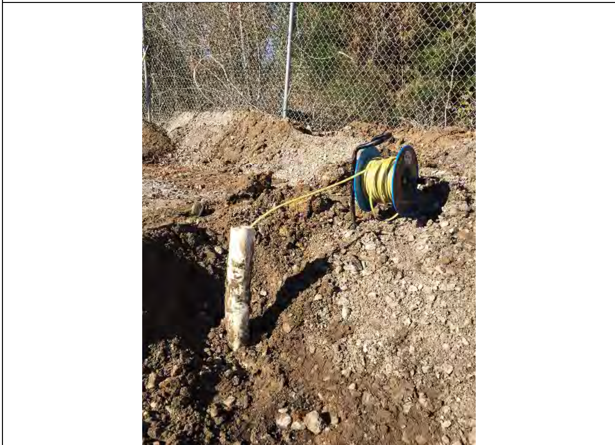
Photo 4 of 12 – Condition of well MW-8 with no well completion and bent casing.
